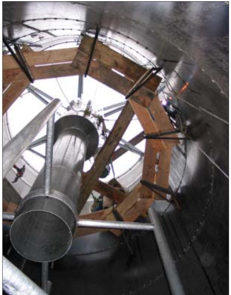
Inside the filter tanks at the Dworshak National Fish Hatchery, welders from R. H. Grover, Inc., make structural modifications to accommodate the new plastic filter beads.
