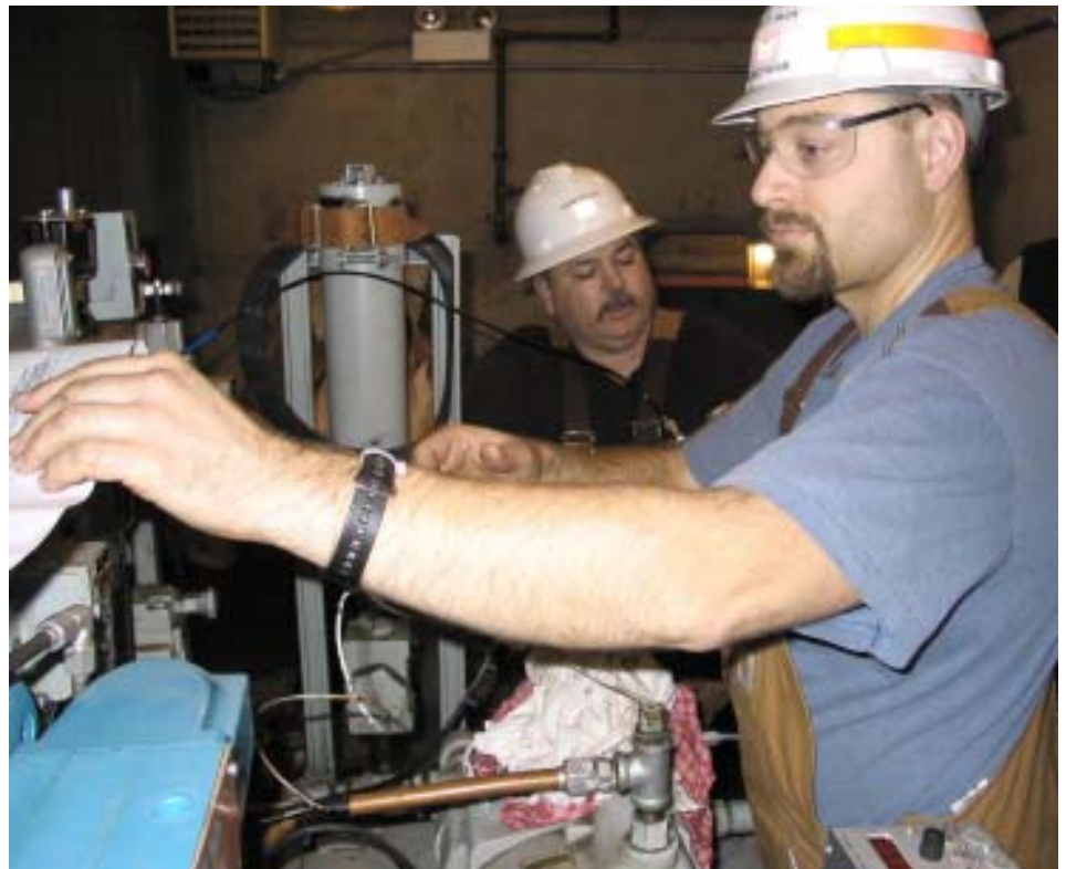
Brett Gillis, power plant electrician, and Norm Rhoads, utilityman, conduct annual maintenance and inspection on the hydraulic unit that opens and closes the navigation lock’s south miter gate.
