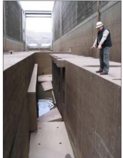
Jim Holston points out the concrete floor slabs on the bottom of Lower Granite Dam’s navigation lock that water has shifted during the past year.
