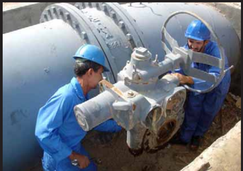
Two Iraqi technicians replace an old valve at one of the intake pipes at the Sweetwater Canal Pump Station #2 located 90 kilometers from Basrah. (USACE Photo)
