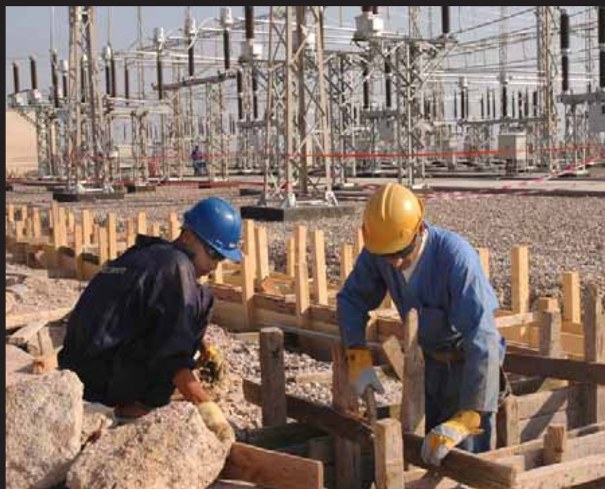
Two Iraqis work on the 33kV cable trench which will help provide permanent power to the Sweetwater Canal Pump Station #2. (USACE photos by A. Al Bahrani)
