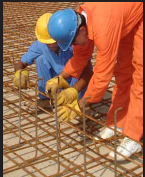
An Iraqi crew prepares the rebar for a concrete pad that will support the fuel storage facility at the Sweetwater Canal Pump Station.
