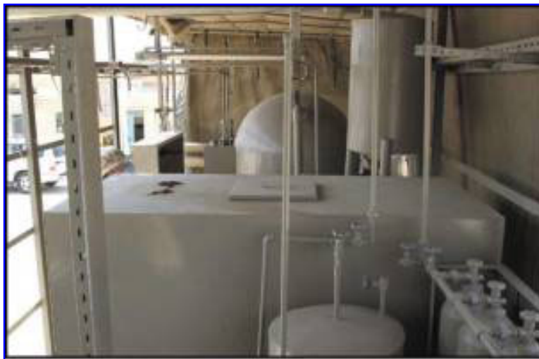
Interior view of fermentor, media tank, water supply tanks, and gas cylinders connected by pipes.
