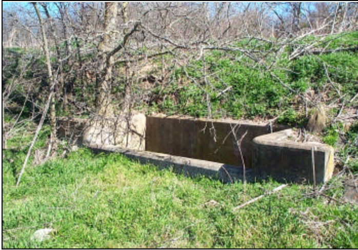
DATE: May 02 DIRECTION: Northwest TAKEN BY: D. Lindsay DESCRIPTION: Old outlet structure at WWTP drying beds
