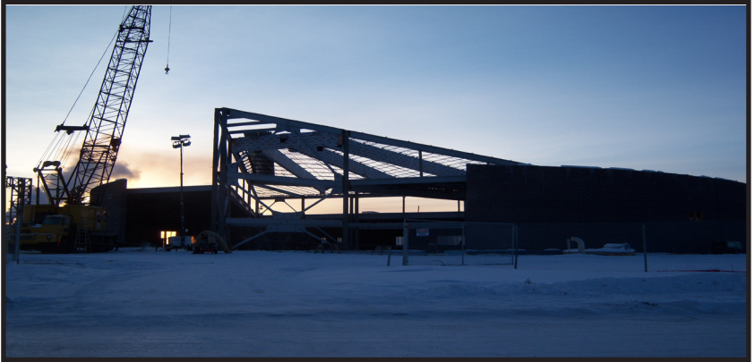
A small business contractor is building a new chapel at Eielson Air Force Base.
