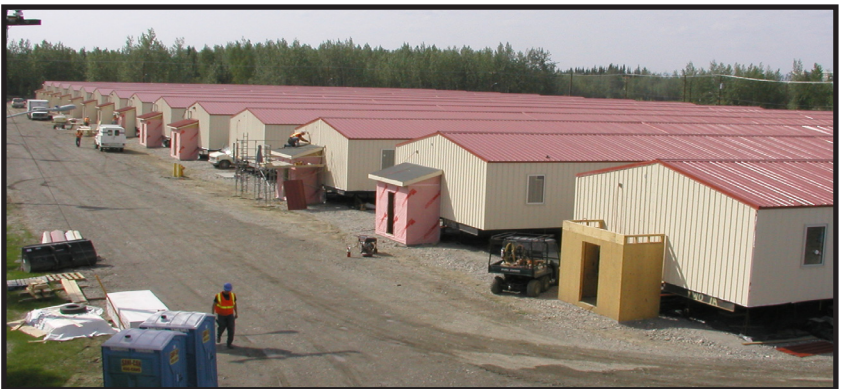
A small business contractor constructed the interim facilities at Fort Wainwright to support the re-stationing of the 4th Battalion, 23rd Infantry Regiment.
