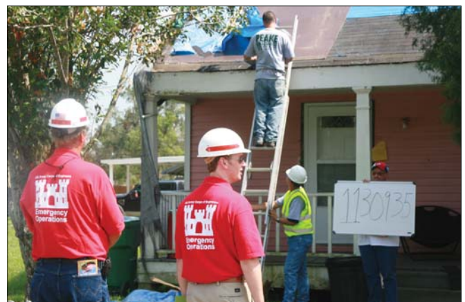
Two Corps' personnel on quality assurance duty inspect a blue roof contracting crew in covering a residential roof in La Place, La., September 7.
