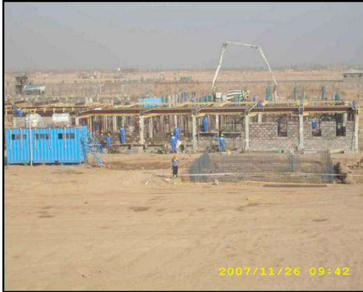
Barracks Construction at the Regional Logistics Center northeast of the ISAF Airfield in Herat.
