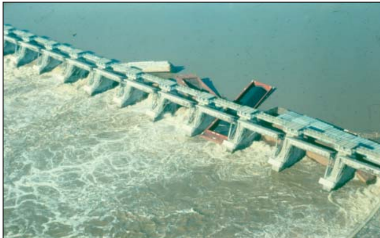
Barges slammed into the Wilbur D. Mills Dam damaging four tainter gates.
