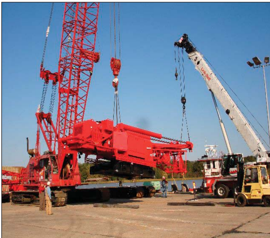
The crane arrived at dawn. It took eight semi trucks to deliver all of its parts. This photo shows the crane following assembly.
