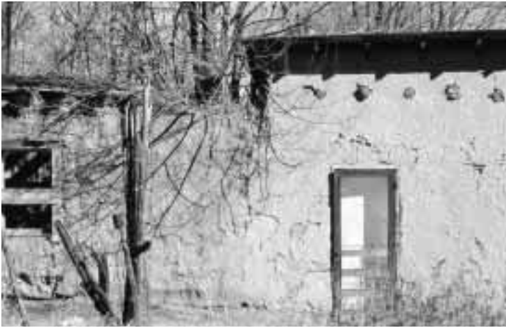
Deteriorating adobe buildings, Taos County, New Mexico. Photo courtesy New Mexico State Monuments, Museum of New Mexico.
