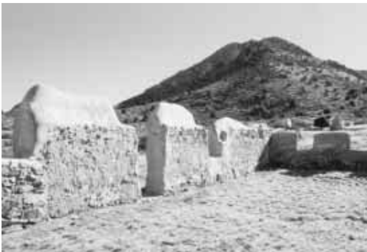
Lime plaster shelter coats over adobe and lime concrete foundation walls of the Cavalry Barracks, Ft. Bowie NHS.
