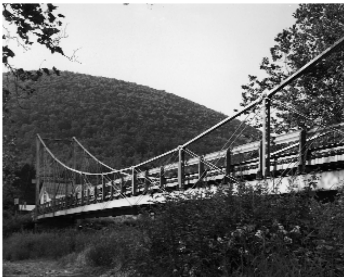
Lower Bridge at English Center, Pennsylvania, showing prominent catenary eye-bar chain and diagonal truss members. Photo by Joseph E. B. Elliott, 1997.
