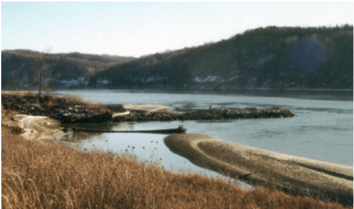
Figure 8a. Notched wing dike, upstream view. Notch is in front of sandbar behind wing dike.
