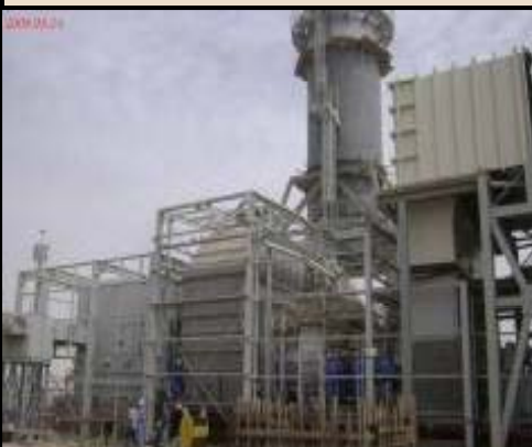
Qudas - Gas Turbine Generator #9
