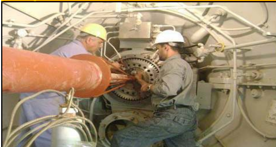
Qudas -Unit 9 auxiliary package alignment final adjustments
