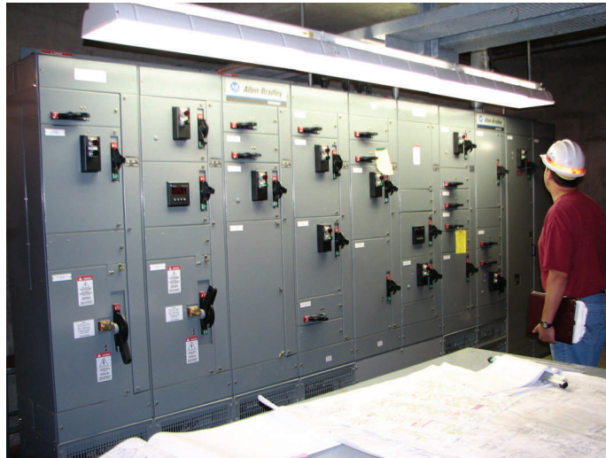
AN EIT EXAMINES AN ELECTRICAL BREAKERS AT COUGAR DAM, OREGON
