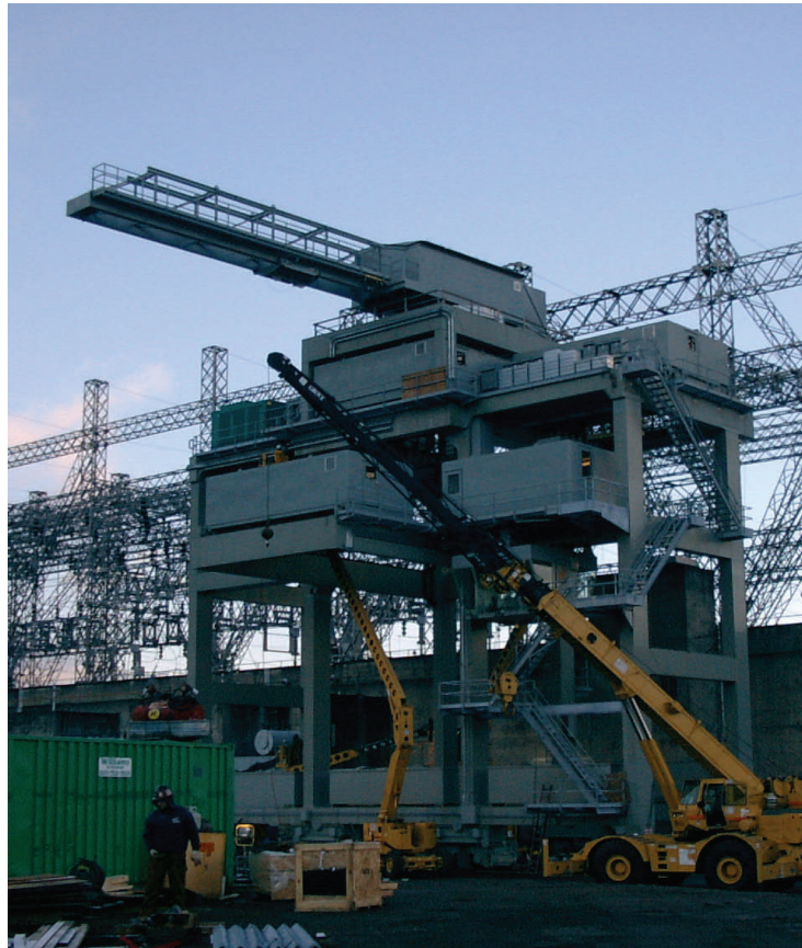
THE 480 TON INTAKE GANTRY CRANE AT BONNEVILLE FIRST POWERHOUSE, OREGON
