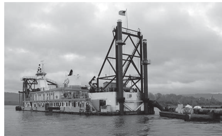
The dredge Oregon clears a channel 400 feet wide, 24 feet deep and half a mile long in the lower Cowlitz River. Photo by Jennifer Sowell.
