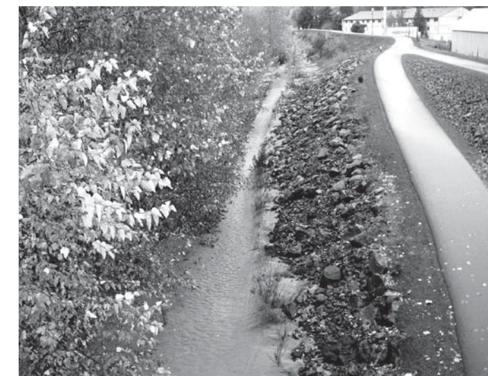
The river deposits sediment between the trees and the levee, resulting in a loss of channel capacity.
