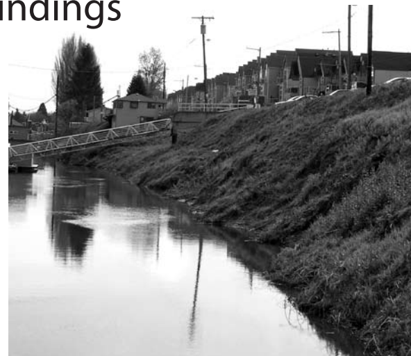
The Bridgeton levee on the Columbia River is threatened by large trees and vegetation.
