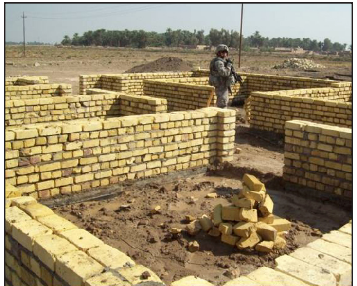
A Coalition Soldier stands amidst the foundation for one of the new schools to be built in the Qadisiyah province.
