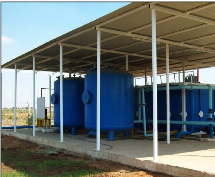
A new water treatment unit will be used to provide clean drinking water to the people in the Qadisiyah province.
