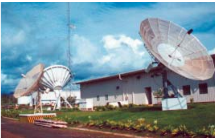
Satellite antennas outside the main transmitter and administration building at IBB's São Tomé Relay Station.
