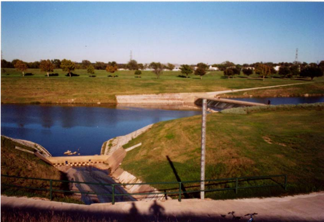
Figure 46. Sump structure located next to Rick's Dam on the West Fork (Property Number 104).
