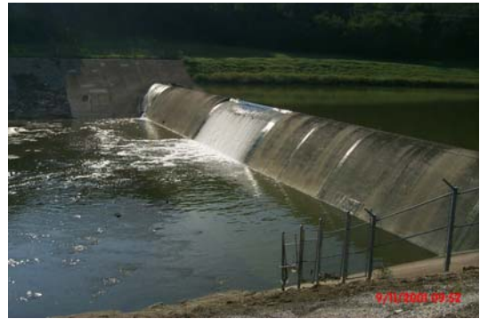
Low water dam in the main channel just east of the Main Street bridge.
