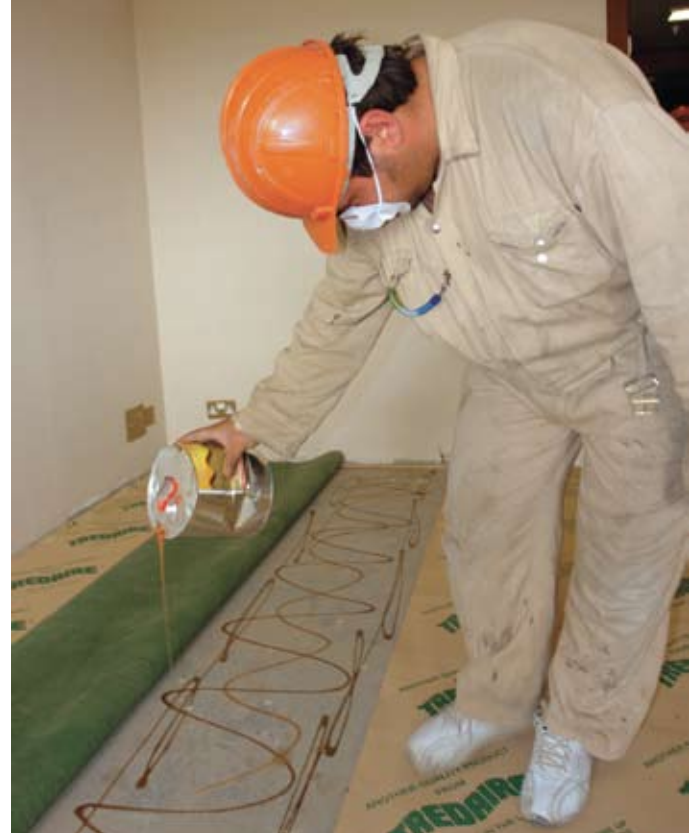
An Iraqi worker pours adhesive for carpet padding as work nears completion on the final floor.
