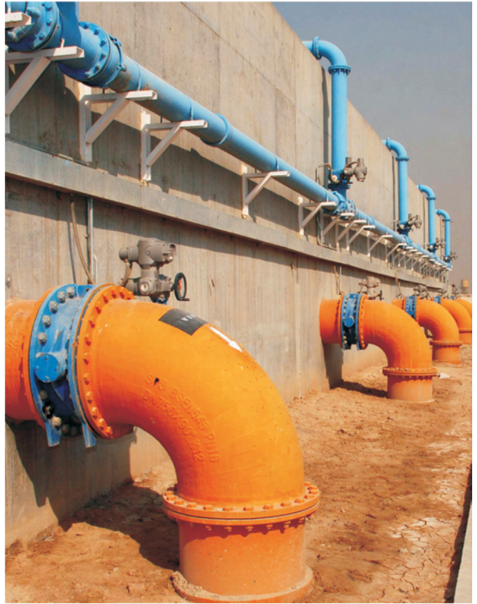
The orange pipes outside the filtration building carry backwash water to keep the filters clean.
