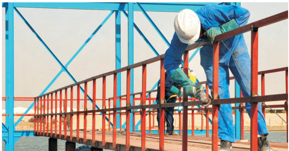
The new steel intake structure is nearing completion at the Qurmat Ali water facility located 9 kilometers north of Basra.
