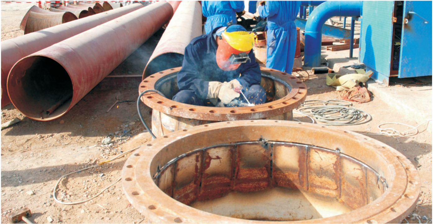
An Iraqi worker welds a new pipe joint at the Qurmat Ali water facility near Basra.
