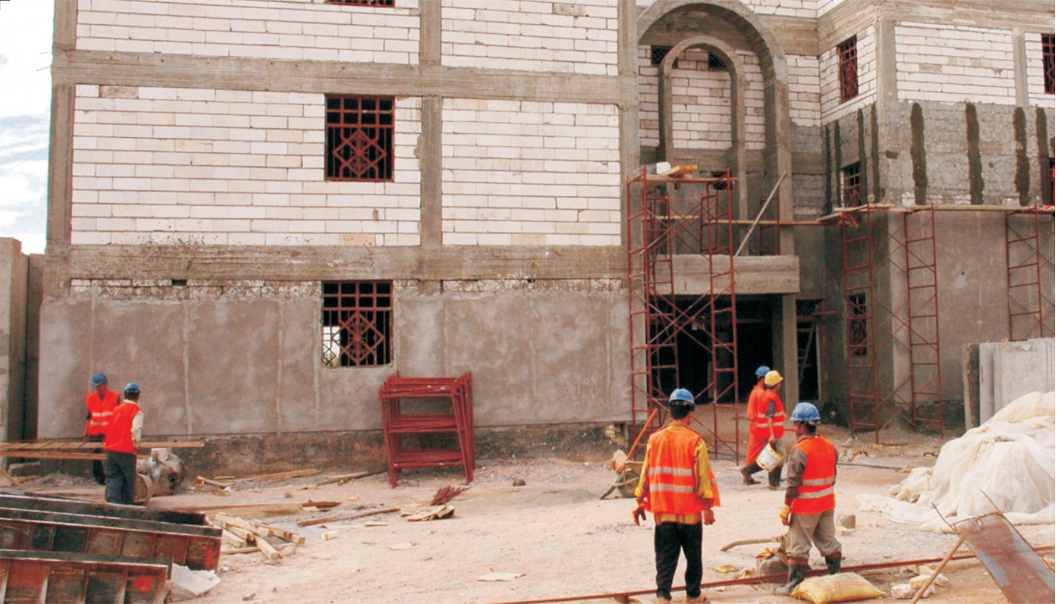
The local Iraqi construction crew is making progress on the new Shatt al-Arab Courthouse in al-Tonoma, Basra Province.
