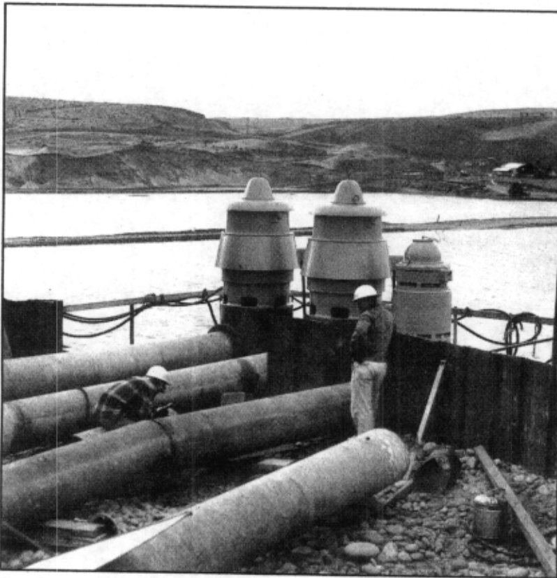
Installation of south shore cofferdam pumps used to keep work area dry during dam construction, December 1956.
