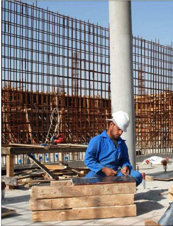
The 3,000-cubic-meter ground storage tank is taking shape at Qurmat Ali water facility located 10 kilometers north of Basra. [USACE Photo by A. Al Bahrani]
