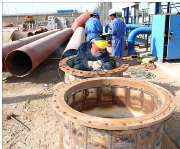
An Iraqi worker welds a new pipe joint at the Qurmat Ali water facility near Basra. [USACE Photo by A. Al Bahrani]
