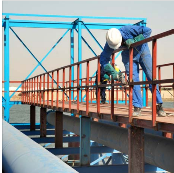
The new steel intake structure is nearing completion at the Qurmat ali water facility located 9 kilometers north of Basra. [USACE Photo by A. Al Bahrani]
