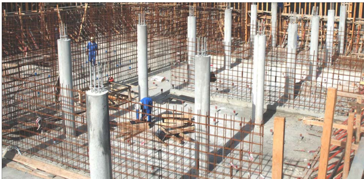
The 3,000-cubic-meter ground storage tank is taking shape at Qurmat Ali water facility located 10 kilometers north of Basra. [USACE Photo by A. Al Bahrani]
