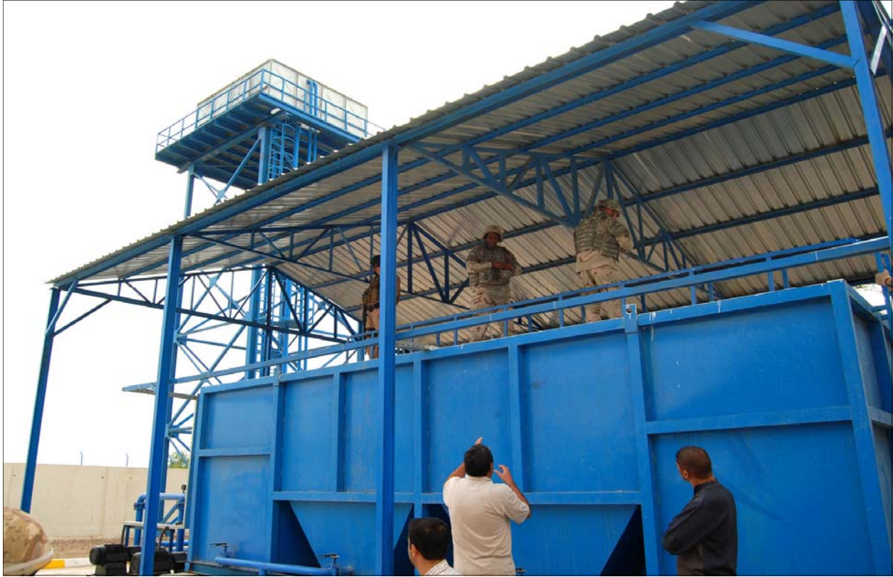
Al Shofa's 50-cubic-meter-per-hour water treatment facility is nearing completion in a rural area north of Nasiriyah in Thi Qar Province. (USACE photo by Norris Jones)
