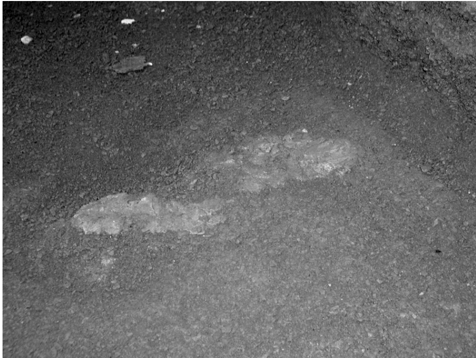
FIGURE 20. CLAY SUBGRADE PENETRATING INTO P-154 SUBBASE ON THE SOUTH SIDE (FOUR-WHEEL TRAFFIC PATH)
