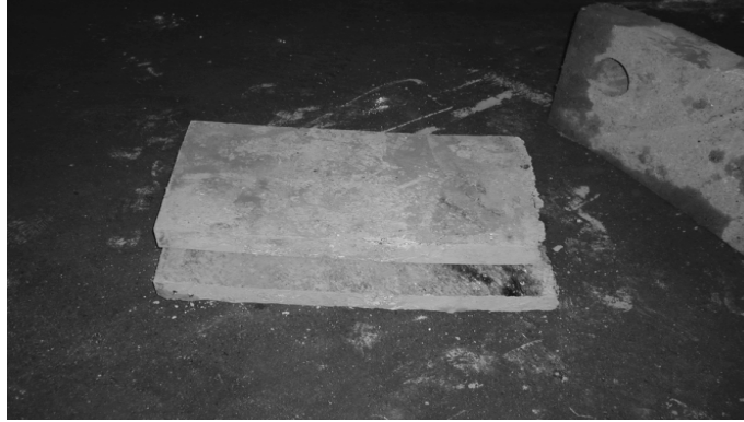
FIGURE 8. P-401 SURFACE EXHIBITING DELAMINATION
