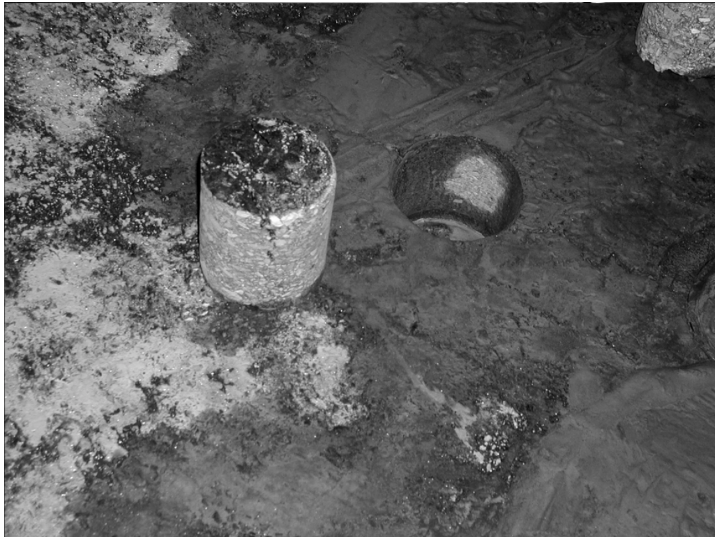
FIGURE 7. P-401 CORE SHOWING CRACK LOCATION
