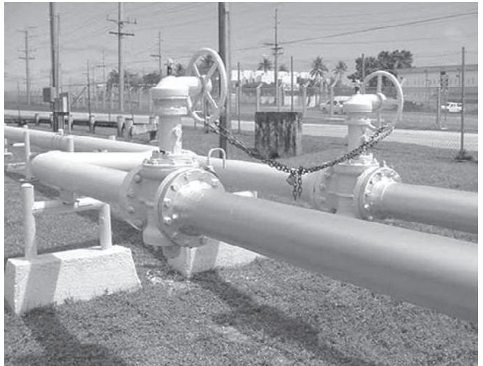
Fuel transfer pipeline.
