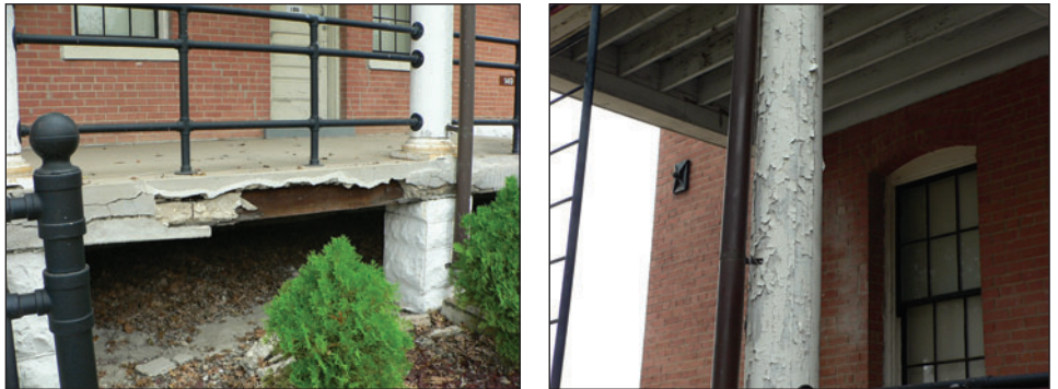
Figure 3: Deteriorated Barracks Building at Fort Sam Houston
