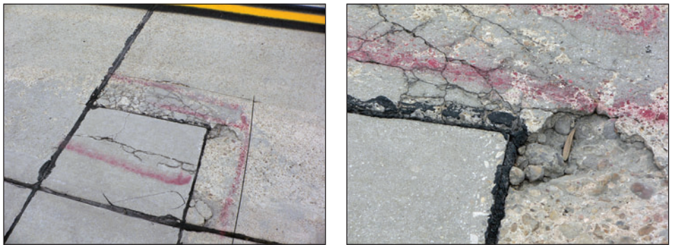
Figure 7: Cracking Aircraft Aprons at Randolph Air Force Base
