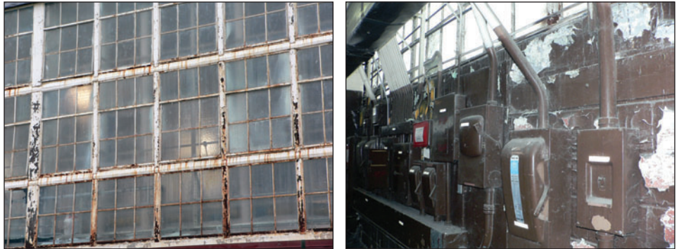
Figure 6: Leaking Windows and Electrical Panels that Created a Safety Hazard at a Deteriorated Aircraft Maintenance Hangar on Randolph Air Force Base
