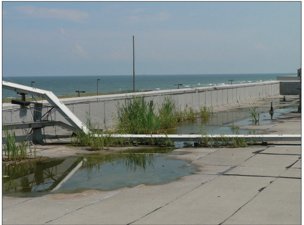
Figure 4: Standing Water on a Leaking Roof of a Weapons and Radar Training Building at an Oceana Naval Air Station Annex
