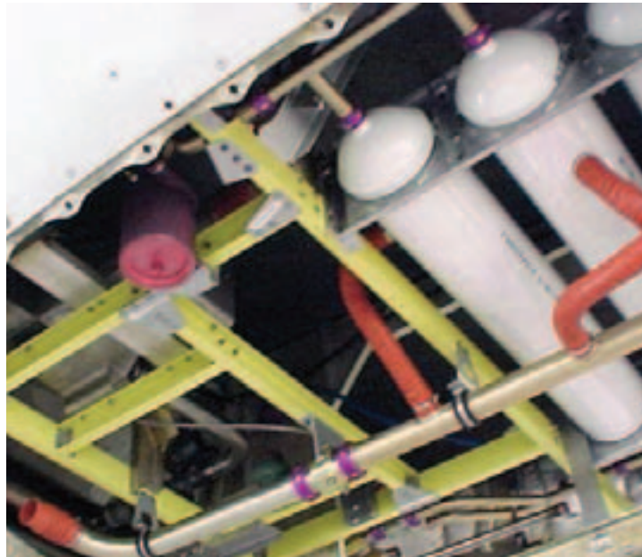
VIEW OF THE FUEL TANK INERTING FROM THE UNDERSIDE OF AIRCRAFT
