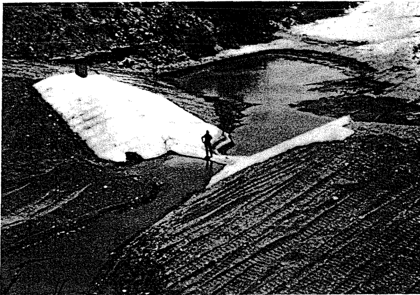
FIGURE 8.—Critical flow flume originally installed for flow measurement at the Walnut Gulch Watershed outlet, 1954.
