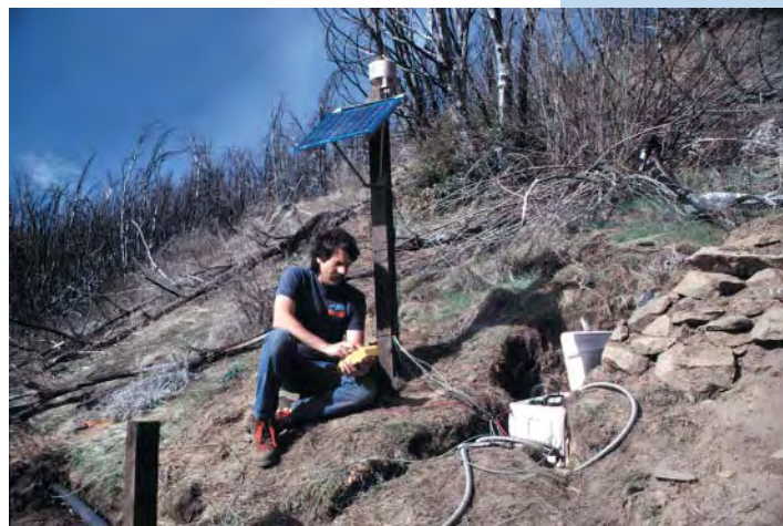
Figure 8. Testing a solar-powered radio telemetry system for remote transmission of real-time landslide data. Photograph by Mark Reid, U.S. Geological Survey.
