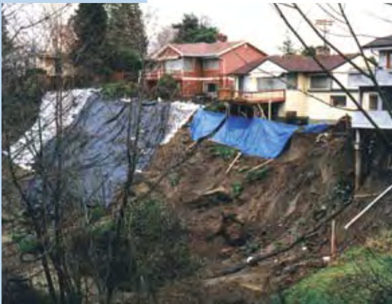
Figure 3. Landslide in northwest Seattle, Washington. Foundation of the house on the right edge of the photograph and the decks of neighboring houses have been undermined. Photograph by Alan F. Chleborad, U.S. Geological Survey.
