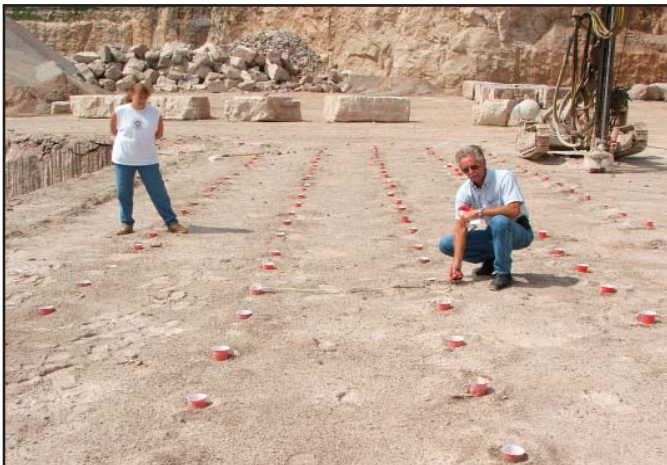
Paper cups mark where holes have been drilled to hold the blasting devices that will cut a section of the rock which will then be cut into the jetty stones.
