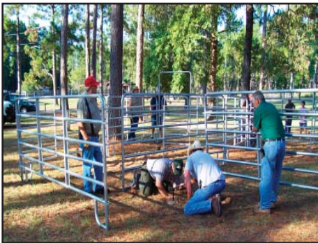
Volunteers and Corps staff rehabilitate the existing horse stalls and hitching posts at Ebenezer Park at Sam Rayburn Lake.
