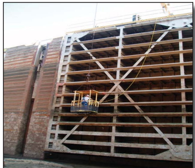
Workers make repairs to the gates of the W.D. Mayo Lock and Dam.
