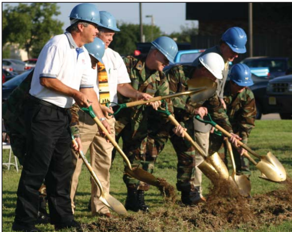
Breaking ground Sept. 13 for the building of the 17th Training Wing Chapel complex are (from left to right) Larry Rogers of the Army Corps of Engineers; Chaplain (Maj.) Michael Goecker; Mike Noret, 17th Civil Engineer Squadron; Chaplain (Lt. Col.) James Ludwikowski, 17 TRW Chaplain; Col. Richard Ayres, 17 TRW commander; 11th District Congressman Mike Conaway and Col. Ada Conlan, 17th Mission Support Group commander.
