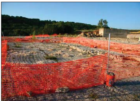
Canyon Lake spillway dinosaur tracks are fenced off and covered to protect them while work is being accomplished on the spillway hardened barrier.
