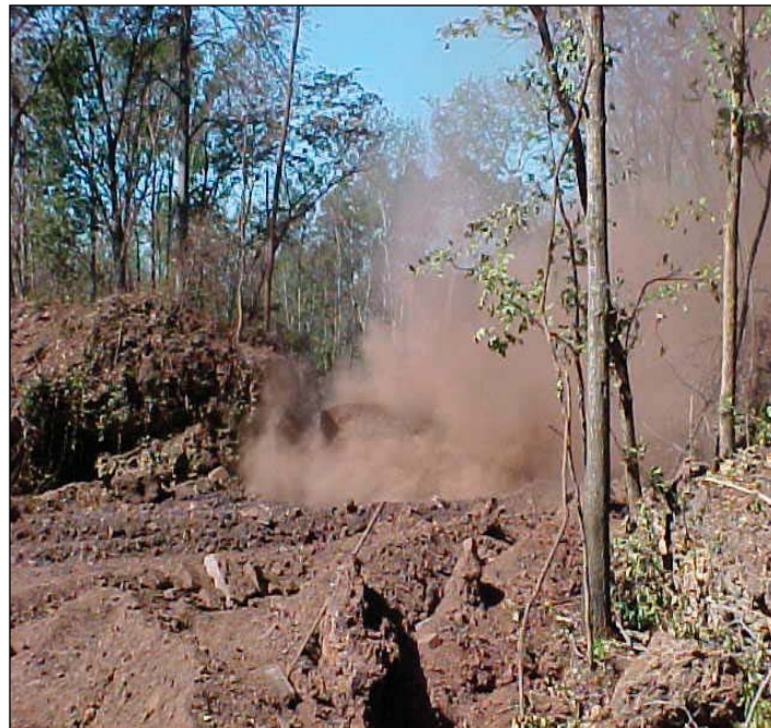
Dust and smoke fly high as work gets under way to extinguish the gob pile fire which has been burning since February.
