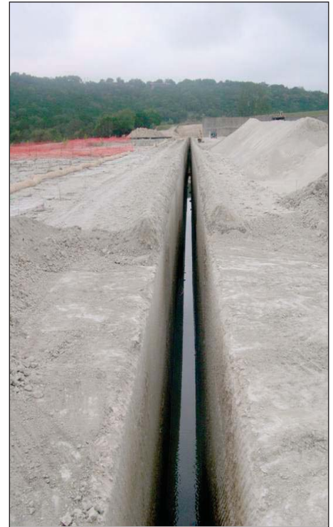
A section of the massive 20-foot-deep by three-foot-wide trench is shown prior to the double steel rebar mats being placed and concrete poured. Photo by James Harvey, Canyon Lake Civil Engineer Technician
