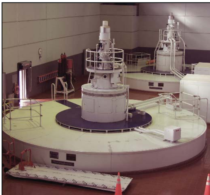
The Powerhouse, which is staffed 24 hours a day, is equipped with two generators each capable of transmitting 25 megawatts of power. (Photo courtesy of Sam Rayburn Project Office).
