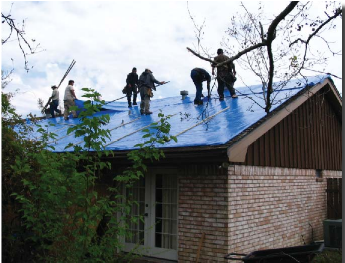
Contractors install a blue roof on a house in Beaumont. Operation Blue Roof is a FEMA-assigned mission of the U.S. Army Corps of Engineers, that provides temporary repairs to roofs in the 22 counties for damage done by Hurricane Rita.
