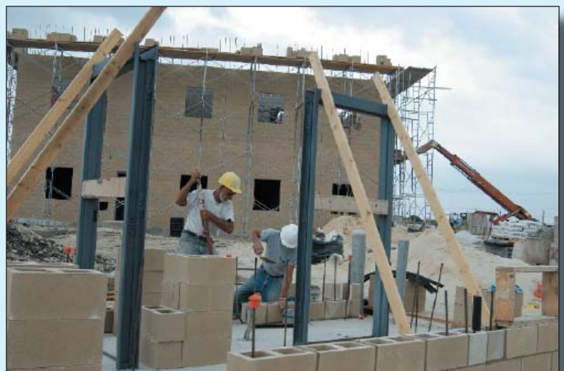
Workers lay blocks for a gate house at the entrance to the mission rehearsal area's training village.
