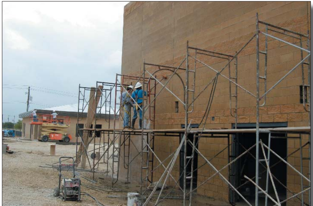
Workers continue construction on a mock bank at an $11 million mission rehearsal area for security forces training at Lackland Training Annex. It also includes a shoppette structure for robbery-type training.
