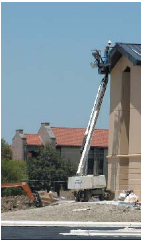
Mel Carter is “finishing out the trim” for the roof of a three-story tech-training dorm nearing completion by Jordan Construction at a cost of $13.52 million at Lackland Training Annex. Carter works for Berbice Corp., a subcontractor.
