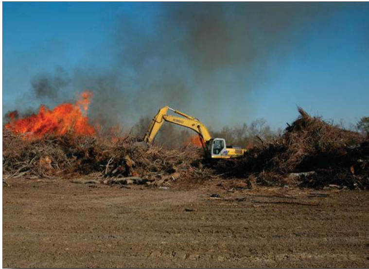
This is not the preferred way to get rid of the debris! Spontaneous combustion lit fires in the piles of debris at the Beaumont Airport debris site.
