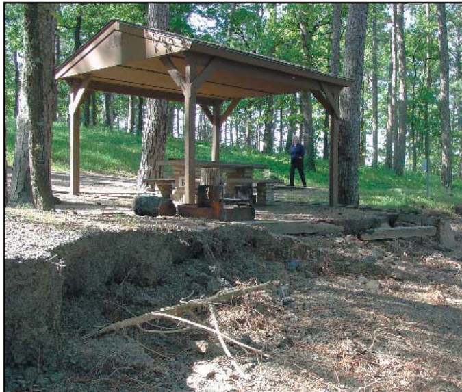
The erosion at this camp site in a Blue Mountain Lake park surfaced as flood waters receded. This type of damage will have to be repaired when funds become available. Photo courtesy of Blue Mountain Project Office.
