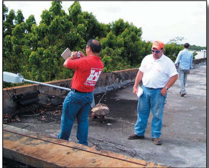
Little Rock Electrical Engineer Tuan Dang takes photos as he and Ozark Powerhouse Construction Representative Joe Jackson inspect the roof of a building in the Dominican Republic during their recent FEST-A deployment to support joint military exercise Beyond the Horizons . Photo courtesy of the FEST-A.
