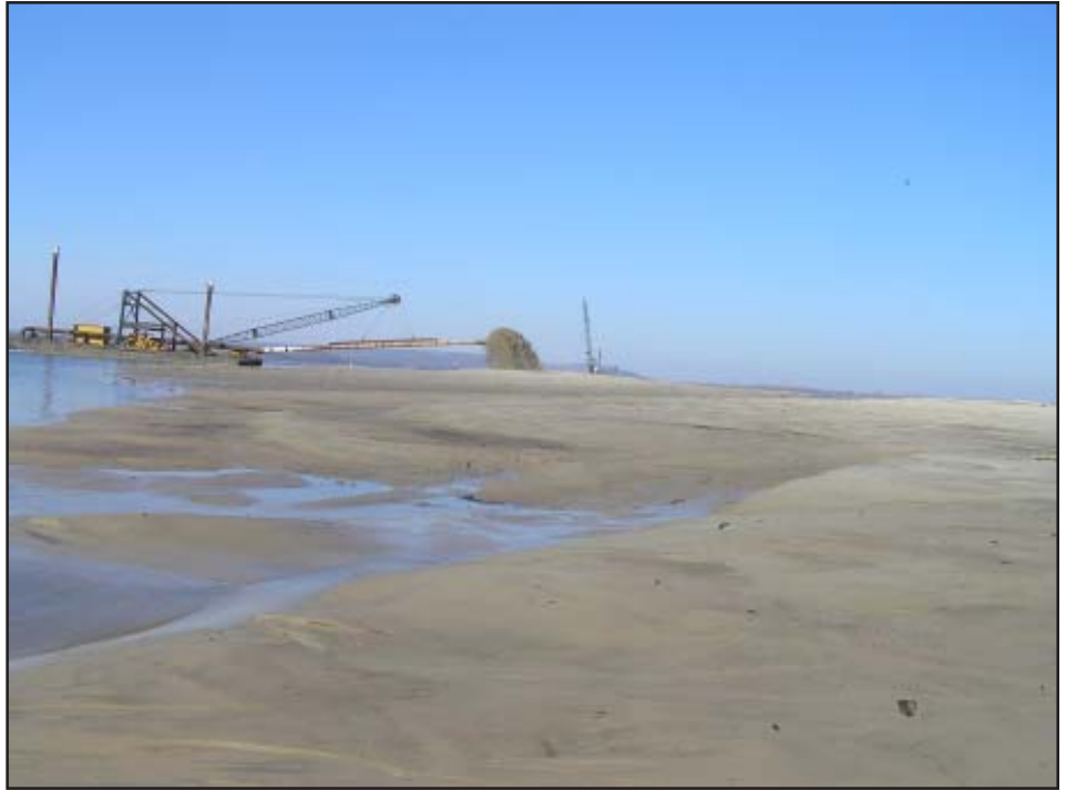
During construction of the 15-acre island. It was built with dredged material made available as the navigation channel was increased from a 9- to a 12-foot depth.
