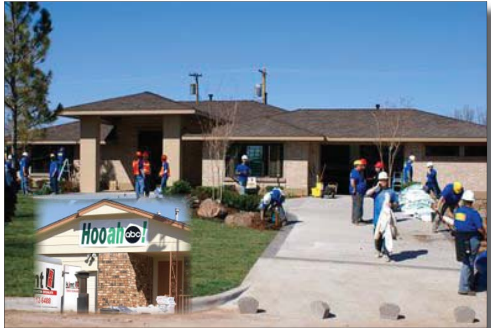
Volunteers work to put the finishing touches on the Westbrook house. Inset: The community shows support for Extreme Makeover and its volunteers.
