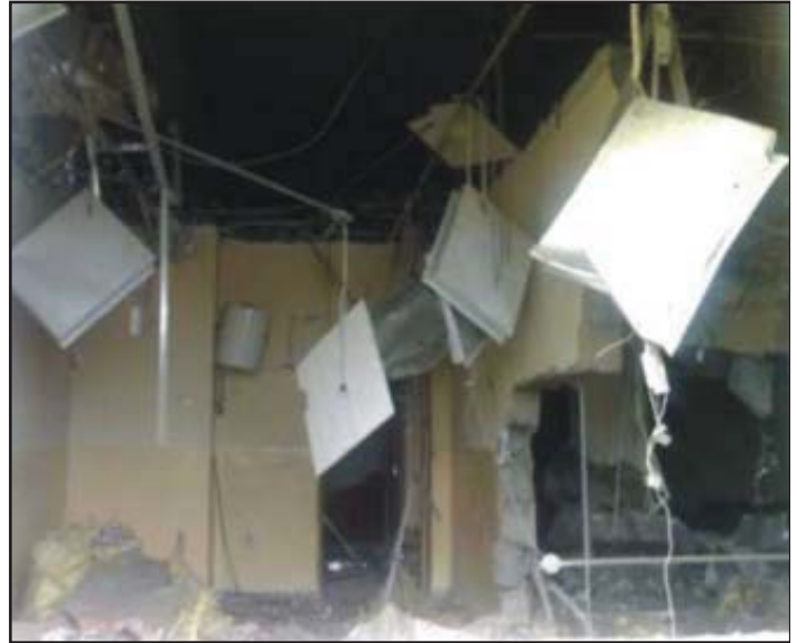
Damages in suspension false ceilings of the Public Health Clinic.
