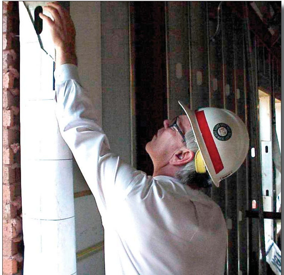
Rod Garner, an assistant area engineer for the Central Arkansas Area Office, inspects the metal studs March 29 at the Child Development Center under construction at Little Rock Air Force Base. Garner recently earned Little Rock District's Engineer of the Year Award for 2007. U.S. Army photo by Steve Ring, Little Rock District.
