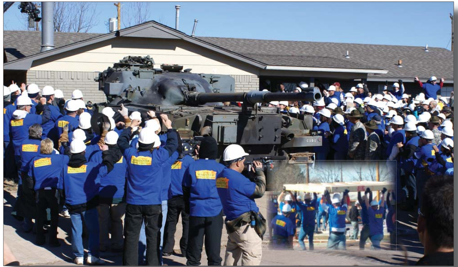
Volunteers cheer as a tank prepares to demolish the Westbrook home, clearing the way for construction to begin. Inset: Volunteers move a prefabricated wall during the construction phase.
