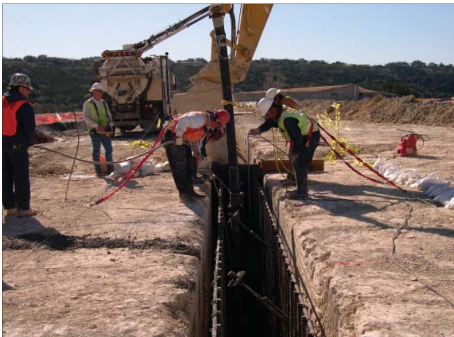
Backhoe Bob’s Excavation contractors prepare to start filling the trench with concrete. The trench measured 20 feet deep, three feet wide, and 1300 feet long. The crew finished the job two months ahead of schedule and with no lost-time accidents. Backhoe Bob’s Excavation received the Fort Worth District’s 1st Quarter 2007 Subcontractor of the Quarter Award.
