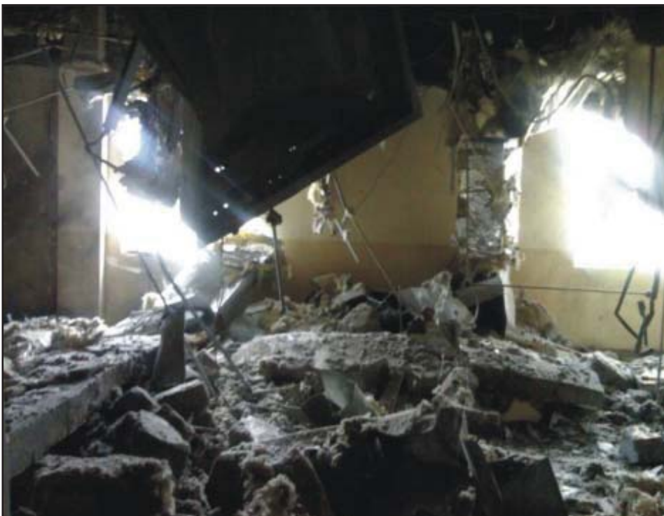
Damage was worse closer to where the bomb was placed.
