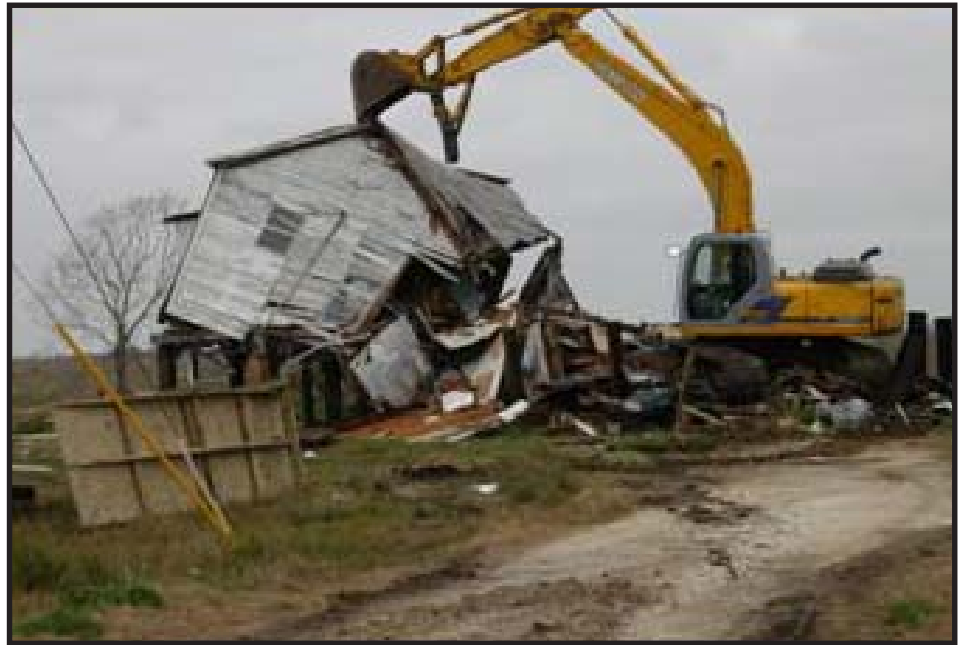
The Federal Emergency Management Agency tasked the U. S. Army Corps of Engineers to demolish 33 condemned houses 13 in Sabine Pass, nine in the City of Port Arthur, and the remainder in Orange County.
