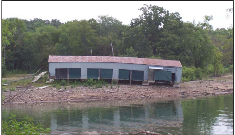
This Tenkiller Lake boat dock was left high, dry, and damaged as the water level receded during the drought.
