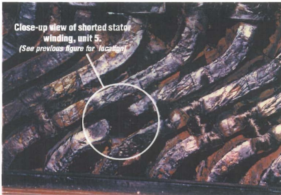
Figure 4-2. Stator Winding Failure Close-Up , Unit 5 (November 1995)
