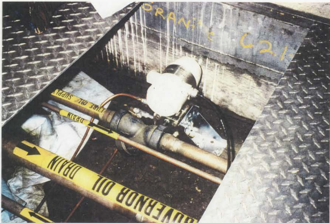
Photo No 5 - Shaft runout measurement using proximity probe. -Lower Granite Dam and Powerplant, Pool Lowering Test, March 1992.
