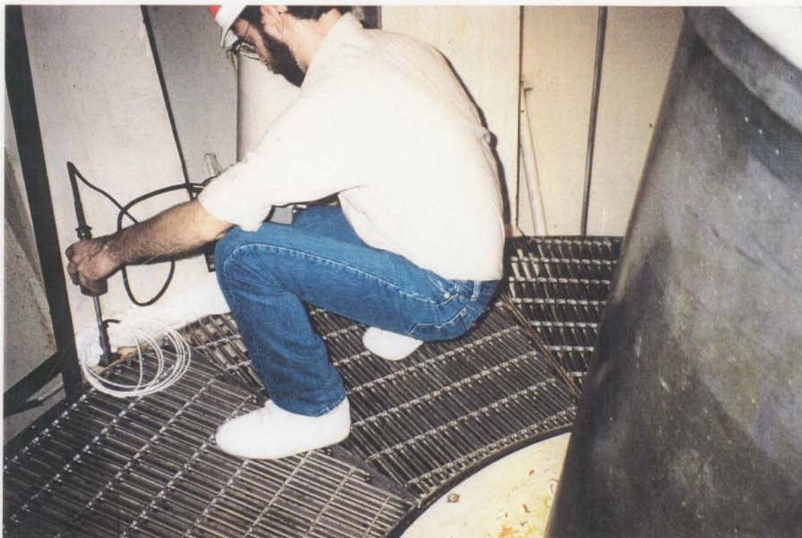
Photo No 7 - Head cover vibration using IRD vibration meter. - Lower Granite Dam and Powerplant, Pool Lowering Test, March 1992.
