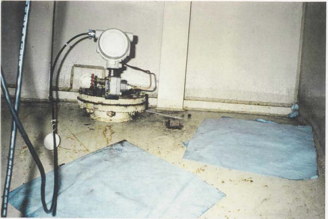
Photo No 9 - Head cover pressure using pressure transducer. - Lower Granite Dam and Powerplant, Pool Lowering Test, March 1992.
