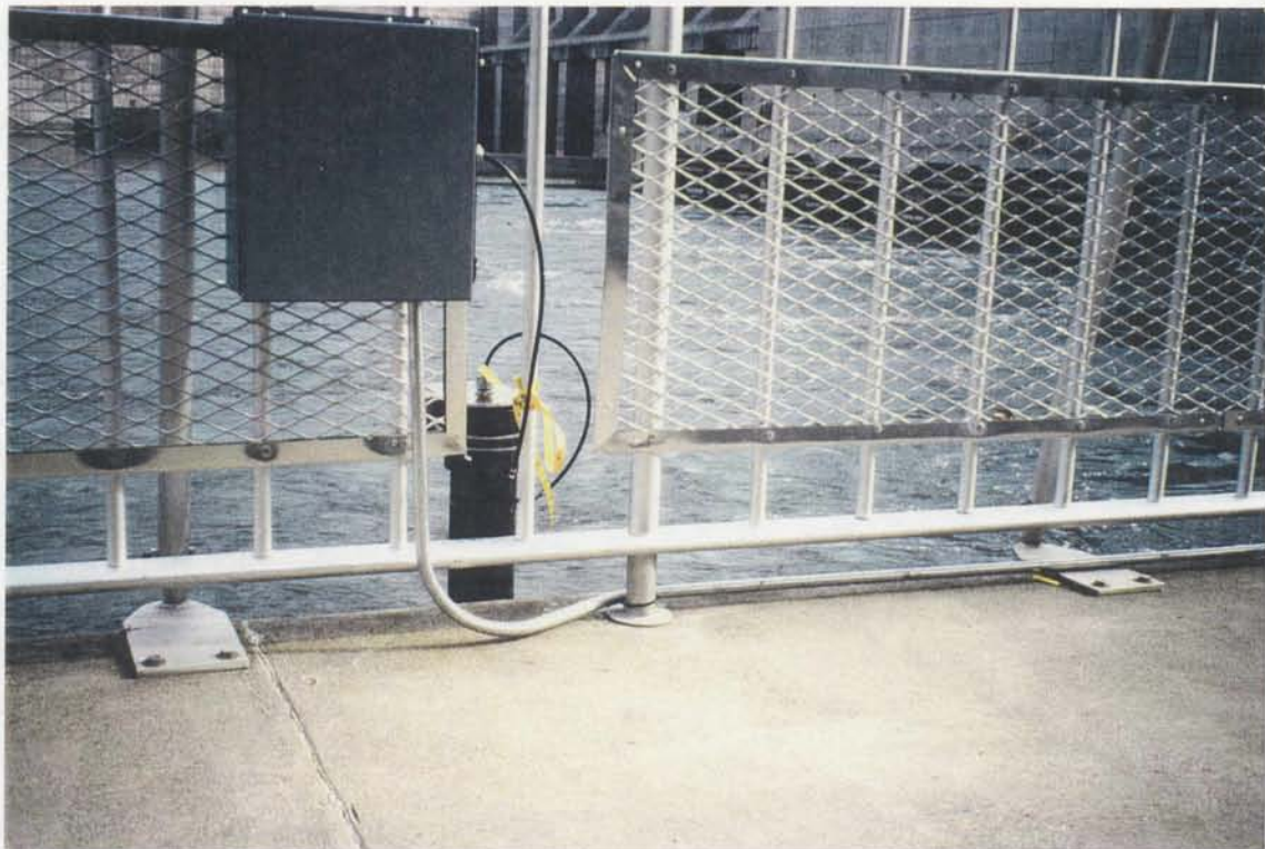
Photo No 2 - Lower water surface using pressure transducer. NEMA enclosure and conduit is part of temporary instrumentation. - Lower Granite Dam and Powerplant, Pool Lowering Test, March 1992.
