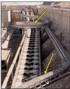
Juvenile Bypass Flume, Lower Goose Dam. Fish are diverted to collection and transport site.
