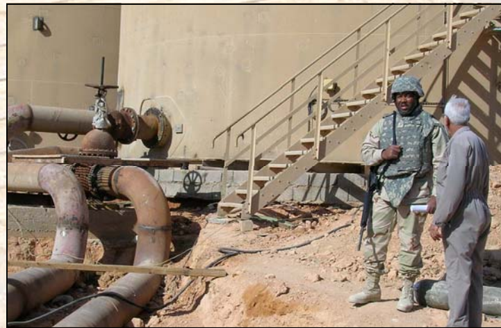
132 kV Mobile Substation and Pump Station at Al Qa'im in Al Anbar Province
