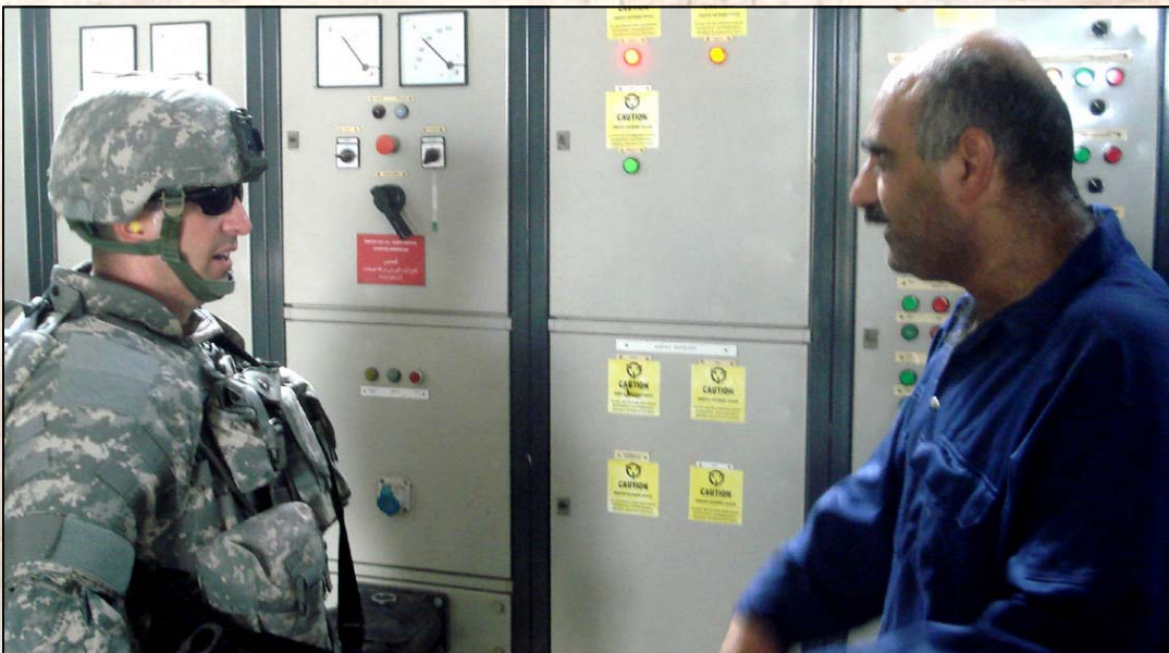
MAJ David Noble checks the new control panel of an electrical substation.
