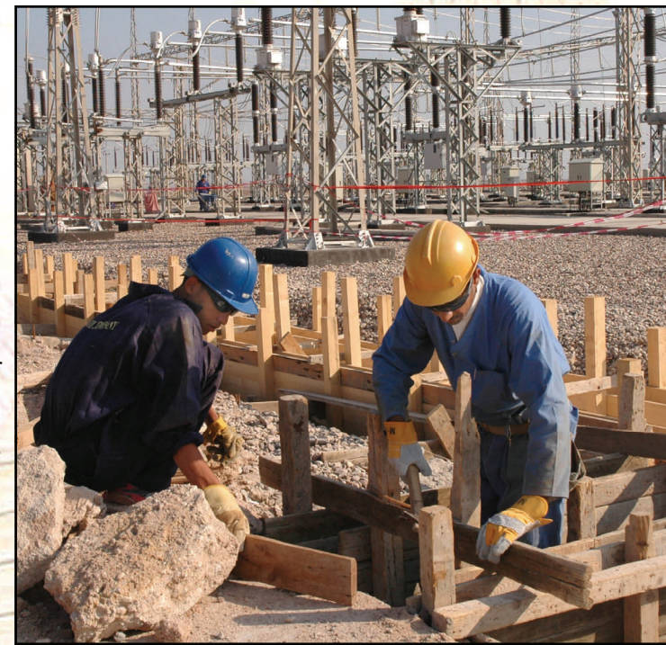
We're connecting permanent power to a pumping station providing Basra its main source of water.
