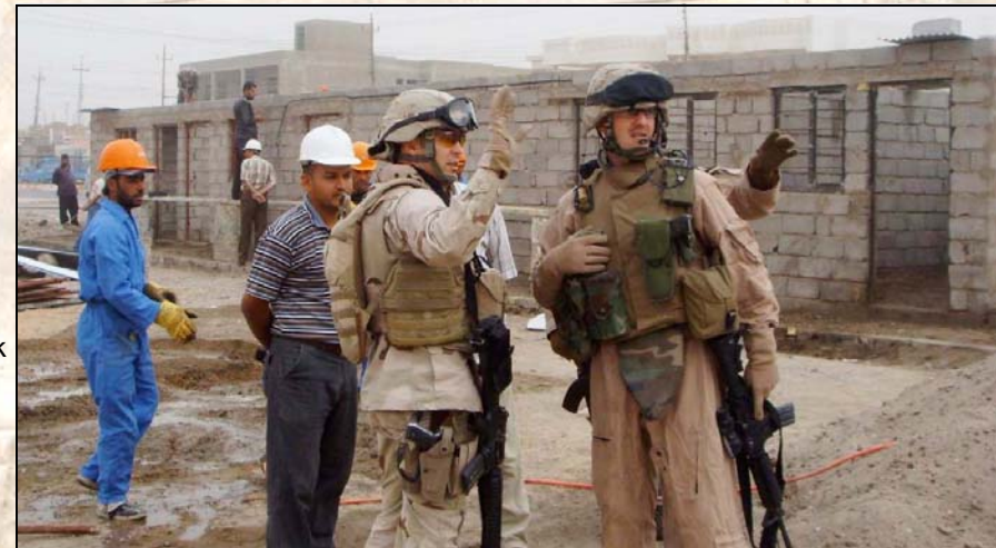
Viewing construction progress at a sewer pump station in downtown Fallujah with members of 4th CAG
