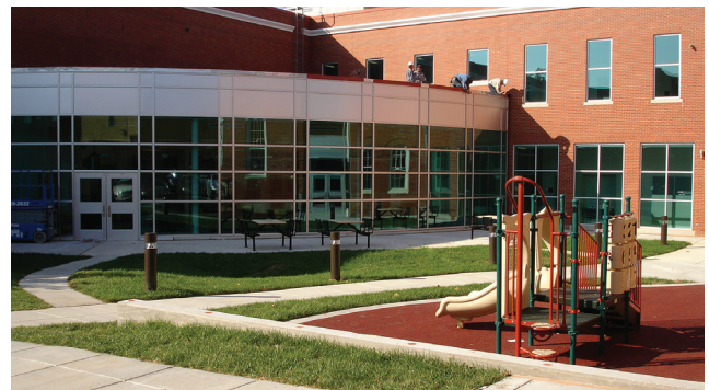
Contractors finish a wall in the courtyard at the Luke C. Moore Academy. In 2006, Baltimore District completed work on the District of Columbia Public School System.
