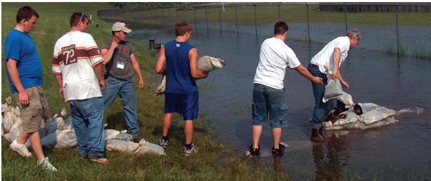
The Corps and county volunteers use sandbags to help repair a damaged levee well after inspection of the levee, floodwalls and pumping stations along the Susquehanna River following heavy rain in June.
