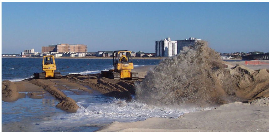
When Lynnhaven Inlet was dredged, the Corps found a beneficial use for the material, placing over 200,000 cubic yards of high-quality sand onto Ocean Park Beach in Virginia Beach, Va. to help protect property from tidal surges and flooding.
