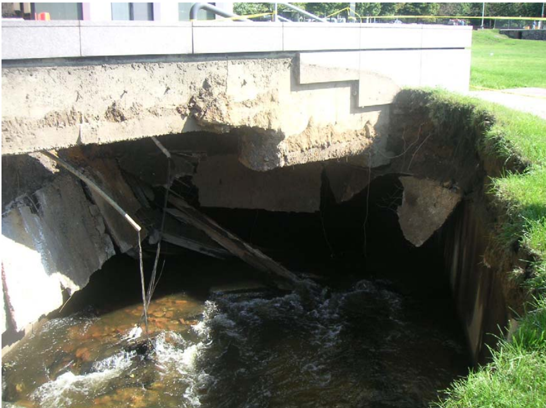
Plate 4. Location of the collapsed culvert roof section.
