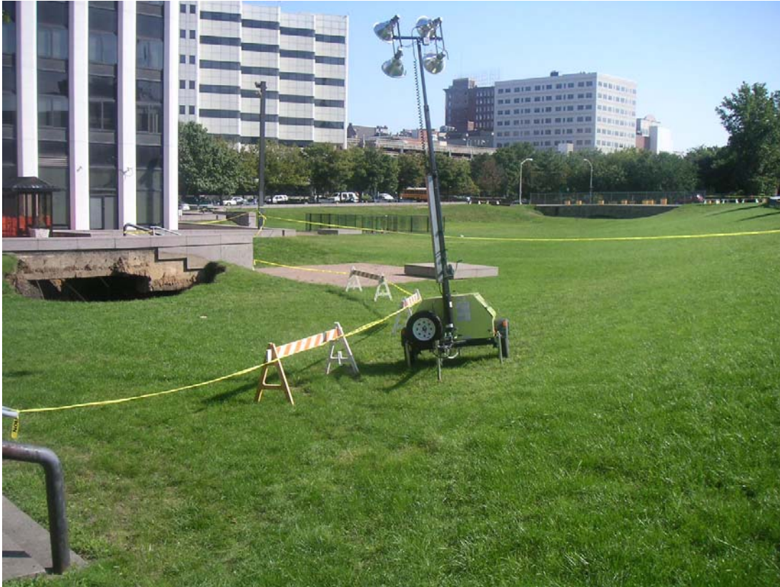
Plate 3. View upstream showing the collapsed culvert roof section.
