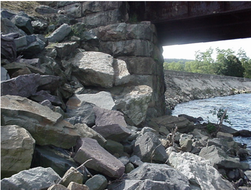
Photo 2. [21 September 2006] Area of loss of riprap immediately upstream of the Railroad Bridge.
