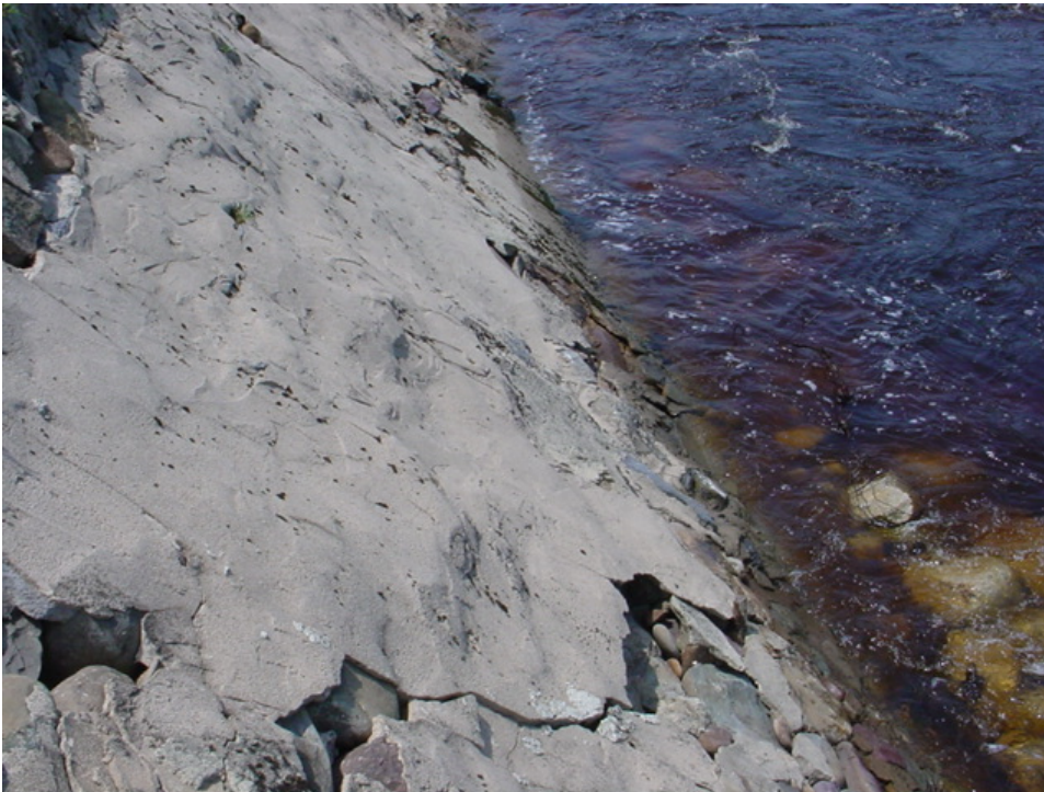
Photo 4. [7 July 2006] Area of deterioration of the concrete facing.
