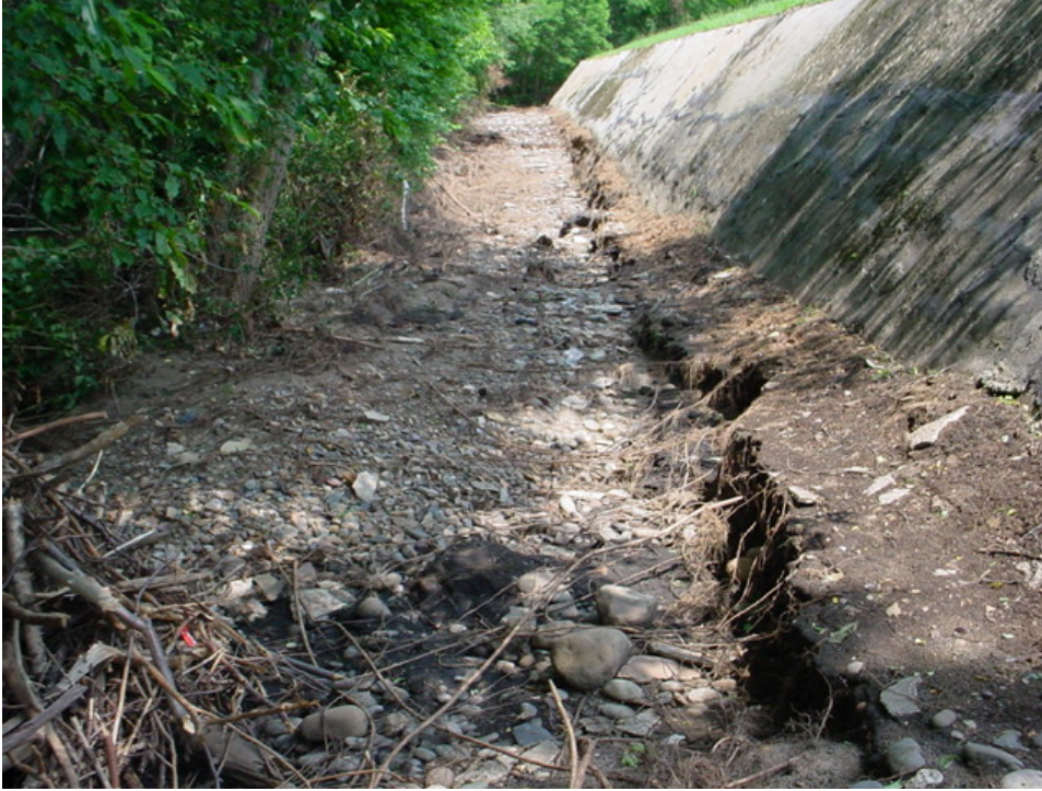
Photo 3. [7 July 2006] Area of erosion of material at the exterior toe of the concrete-faced portion of the levee.
