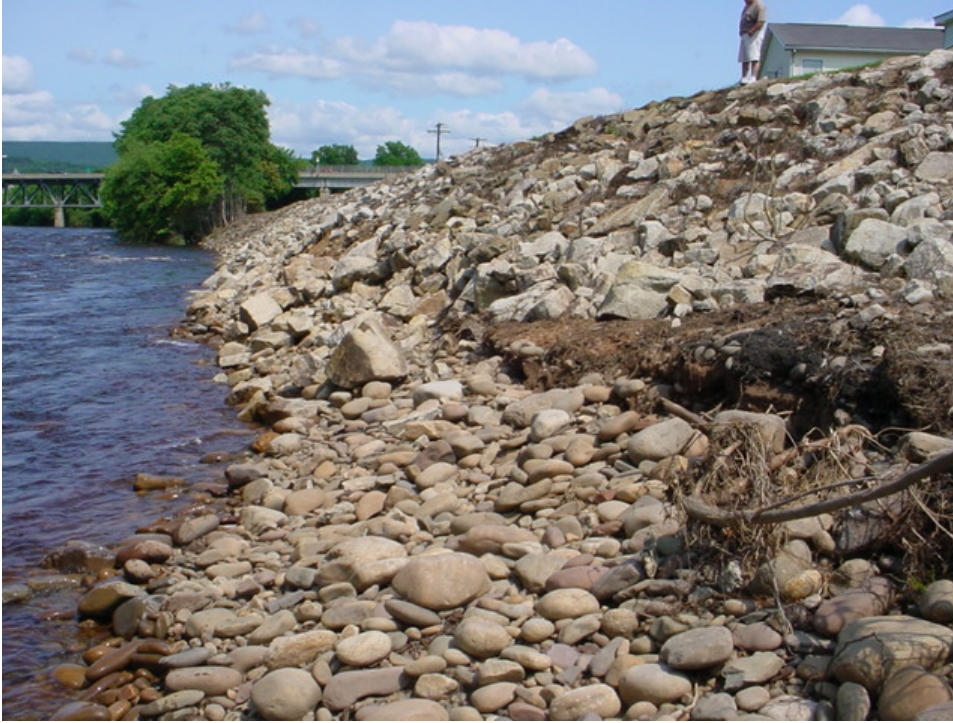
Photo 1. [7 July 2006] Area of loss or sloughing of riprap adjacent to the Borough Hall.
