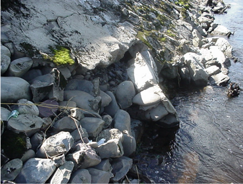
Photo 5. [21 September 2006] Loss of riprap at the toe of the levee below the concrete facing.
