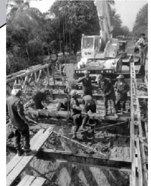
SDF members repairing roads mainly used by local people (Takeo in January 1993)
