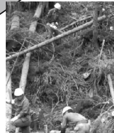
SDF members removing trees that fell due to typhoon in order to prevent secondary disaster (Kusu Town in Oita Prefecture in May 1992)
