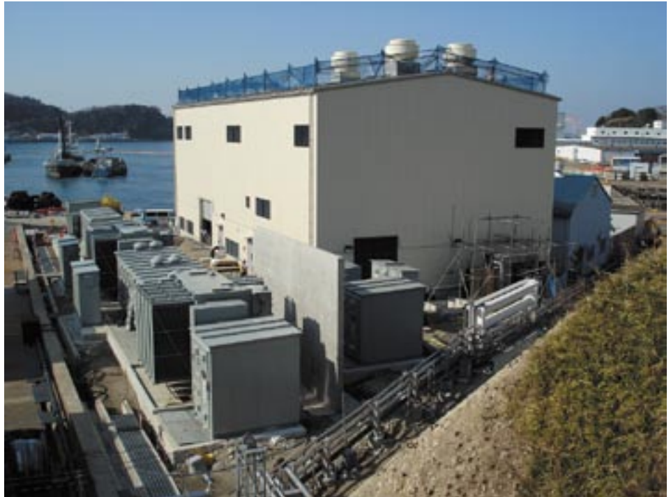
High Quality Water Facility building at Yokosuka Naval Base (P998). U.S. Army Corps of Engineers Photo
