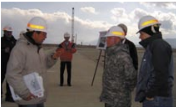
Maj. Gen. Bo Temple gets an update on the runway relocation project at Iwakuni.
