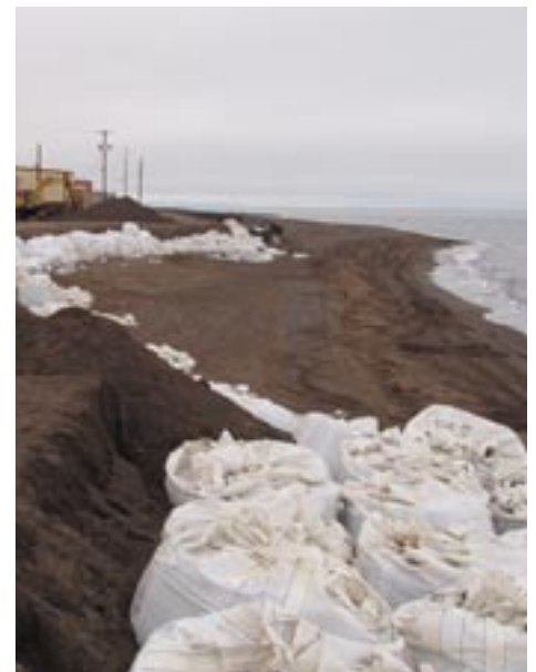
Sandbags were used in an effort to protect the Kivalina shoreline last year. Alaska District Public Affairs photo
